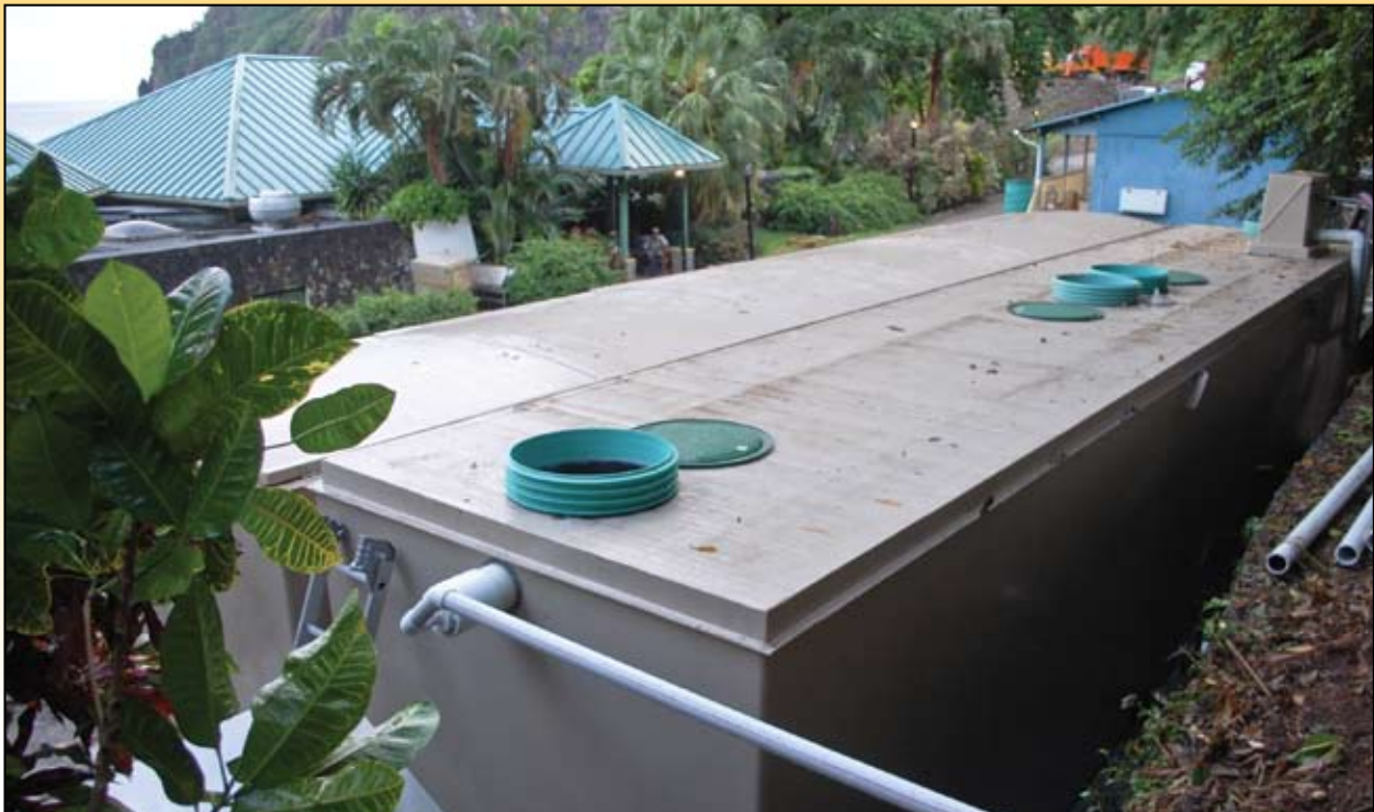
This AX-Mobile was installed on an award-winning, 60-room resort on the island of St. Lucia, in the Caribbean. The AX-Mobile replaced an old activated sludge plant that was destroyed by Hurricane Tomas on Oct. 31, 2010. Orenco was brought into the project on November 18 and had the AX-Mobile wastewater treatment system shipped, installed, and commissioned by the resort's December 20 re-opening date, in time for holiday bookings. The lighter weight of the fiberglass AX-Mobile was important for this island installation, where the equipment to lift a heavy metal package plant wasn't available or feasible for this hilly, volcanic site.
