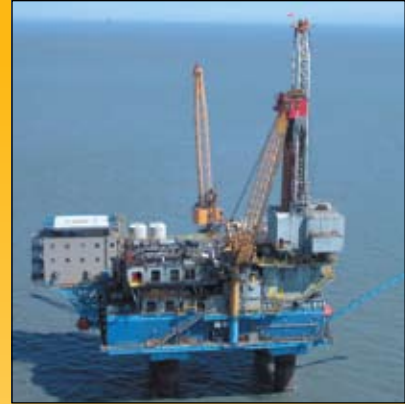
In 2002, the Osprey Oil Platform in Cook Inlet, Alaska replaced an extended aeration plant that couldn't meet permit limits with Orenco's AdvanTex® Treatment System, installed onto a mezzanine.
