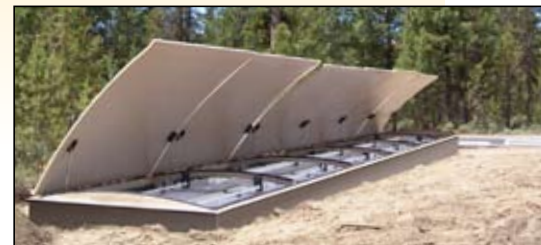
This full-sized AX-Max wastewater treatment system was recently installed at a 50-site campground in the LaPine, Oregon State Park.
